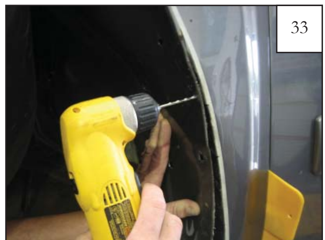
With 3/32" drill bit, drill through mark and the bent tabs of metal behind them for four locations along edge of wheel well.
