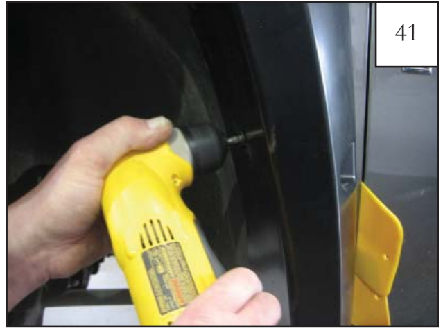
Install Screws (SW1-0056) through flare and into hole in sheet metal in both locations.
