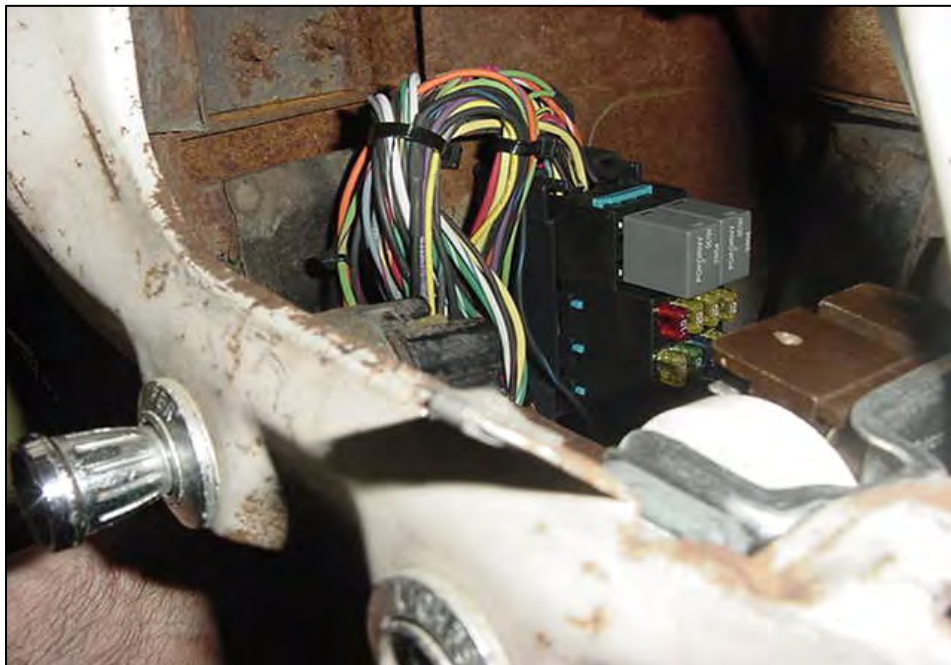
Figure 6-2 Fuse Block Position
