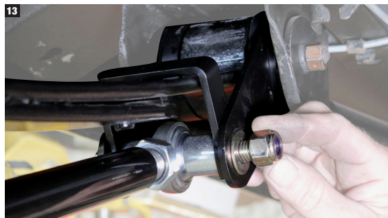
13. Then, slide the front of the traction bar in place and insert the bolt to hold everything together. The top of the anti-torque strap should be flush with the leaf spring
