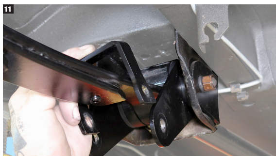
11. Next, slide the anti-torque strap over the top of the leaf spring and line up the bolt holes with the front mounting brackets.
