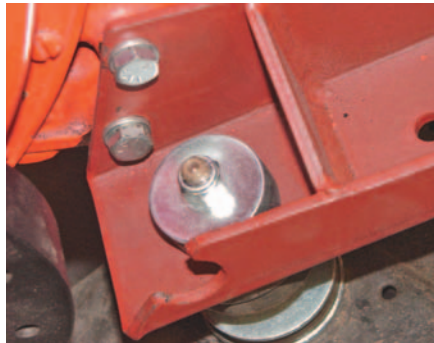
Photo #8: With the pump bracket in place, lower the engine down and install the new upper rubber cushion, washer and nut.
